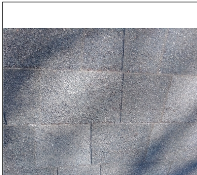
Upclose location with reference to conditions of shingles. (This only reflects the worst location and does reflect all the shingle conditions.)
