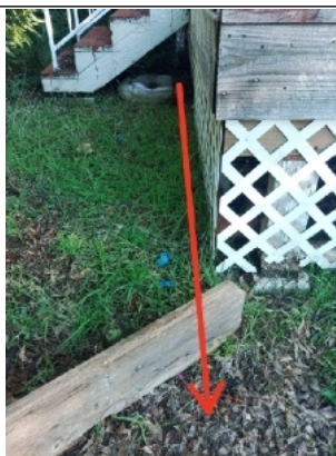
Recommend installing a downspout and attaching corrugated drain extension. Make sure to run past the girder and post members of the deck.
