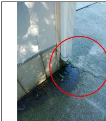
Crack on slab is from excessive water run off from lack of a proper elbow or drain extension.
