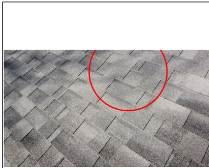
Location shows fiberglass lining around the base of the shingles.
