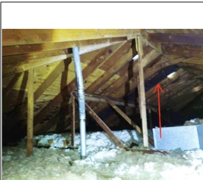
This location is of concern with delamination. Excessive moisture stains are evident on rafter and the arrowed location (referenced in the roof section) is of concern with delamination.
