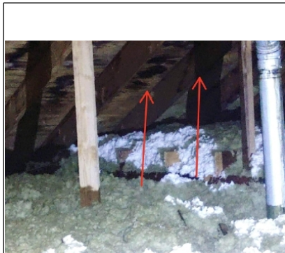
Arrows points to more locations of concern. (Again, at this location, when walking the roof the sheathing was not delaminated) only one small section of sheathing appeared to be delaminated.
