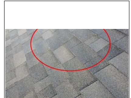
Location shows fiberglass lining around the base of the shingles.
