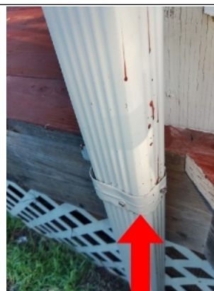
Recommend refastening loose downspout to rim board of deck.
