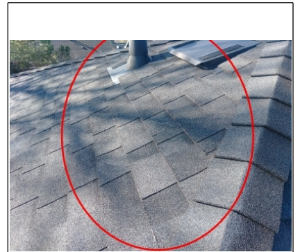
Location shows fiberglass lining around the base of the shingles.
