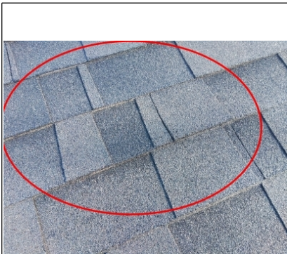
Location shows fiberglass lining around the base of the shingles.
