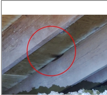
Moisture stains are evident from possible active leak.
