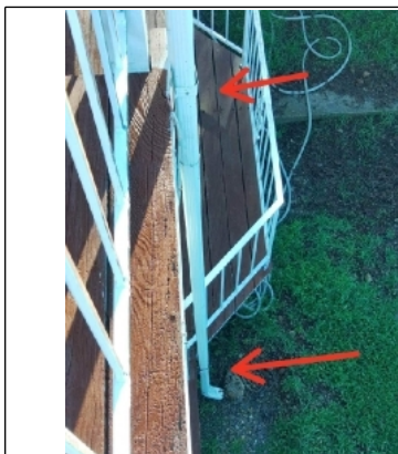
Recommend refastening loose downspout to both rim members of the deck. The lower rim member will need a 1-1/2" thick pressure treated block installed to make the proper attachment.
