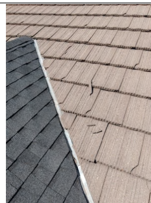
Recommend having cracked and damaged tiles replaced or repaired by a Licensed Roofing Contractor.
