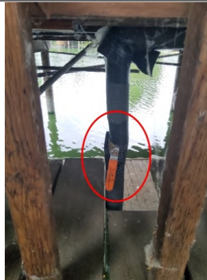
Water shut off valve location
