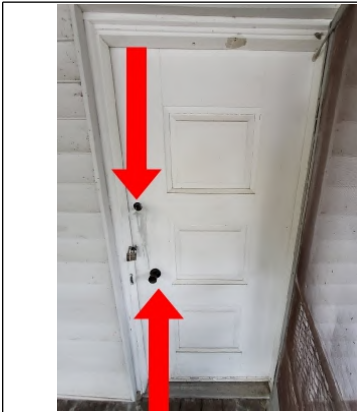
Recommend replacing door handle and deadbolt.
