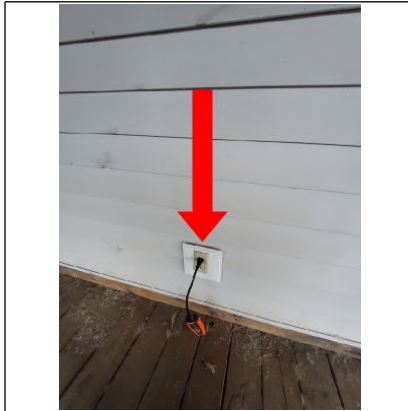
Recommend replacing electrical outlet with a GFCI and installing an exterior cover.
