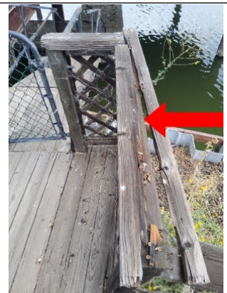
Recommend replacing all top plate members with pressure treated or resistant to wood decay material.
