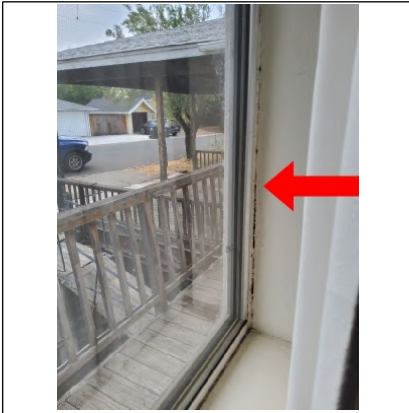
Recommend additional caulking be applied.
