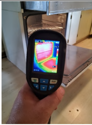
Thermal Imager shows oven properly operates.
