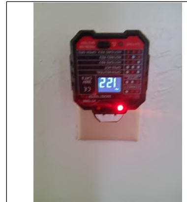
Electrical outlet is not grounded but shows proper operation.
