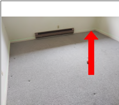
Laser level shows floor has a 1" slope at noted location.
