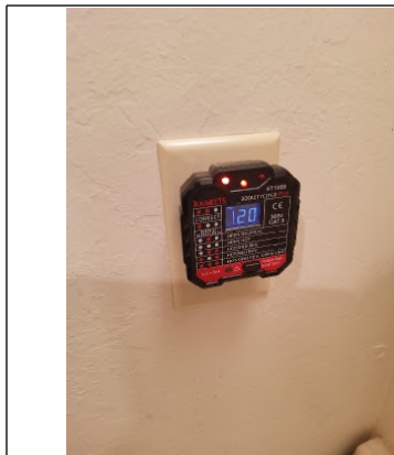
Electrical outlet shows proper operation, grounding and polarity.
