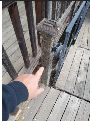
Recommend releveling post and refastening to rim member and installing a galvanized angle bracket.
