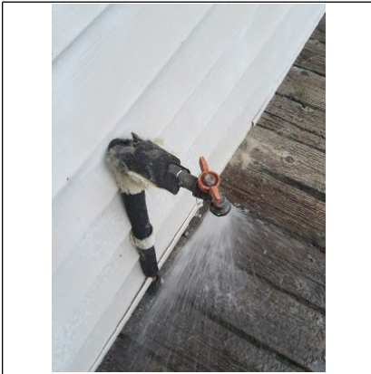
Recommend replacing leaking hose bib
