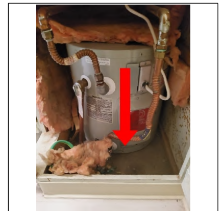
Water heater is in a living area and should have a drain pan. Recommend having a drain pan installed and a drain line stubbed to the exterior wall in the underfloor location. (Or in this situation the floor)
