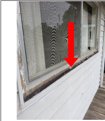
Recommend installing new exterior trim around window and properly painting and caulking.
