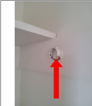
Recommend replacing broken hardware
