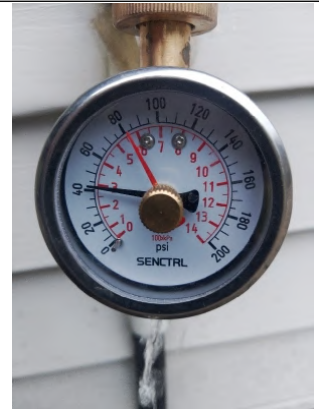
Water at shut off location is 41 PSI which is a satisfactory water pressure. The ideal water pressure for a house is between 40 to 65 psi.
