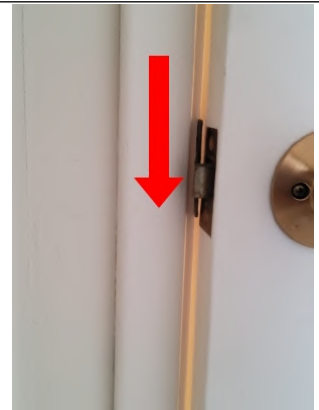
(Reference to prior slide) Recommend moving strike plate down if raising the door slab does not fix the latching issue.
