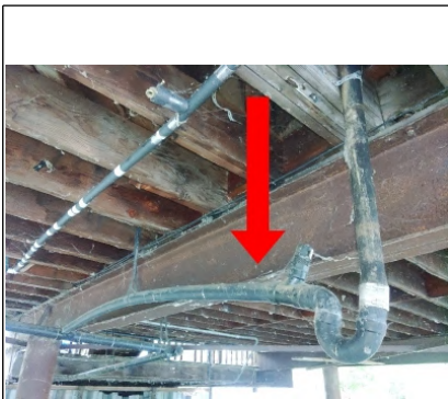
ABS drain line must have a minimum 1/4" fall per ft. Recommend having properly pitched by a Licensed Plumber.
