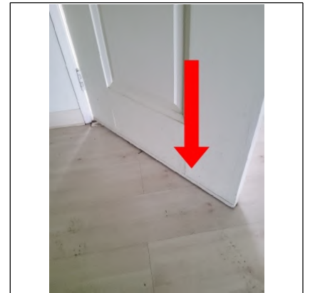
Recommend replacing door sweep to ease the operation of the exterior door.
