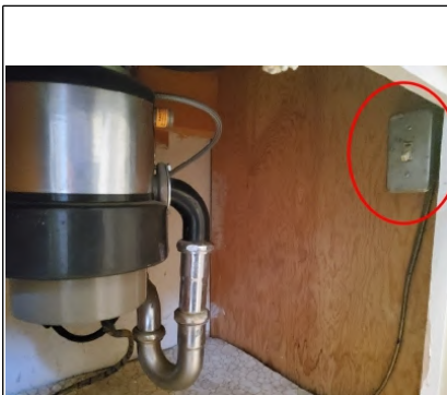
Garbage disposal shows proper operation when testing.
