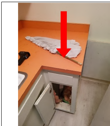
Water heater location
