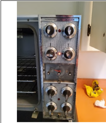
Oven dials show proper operation.
