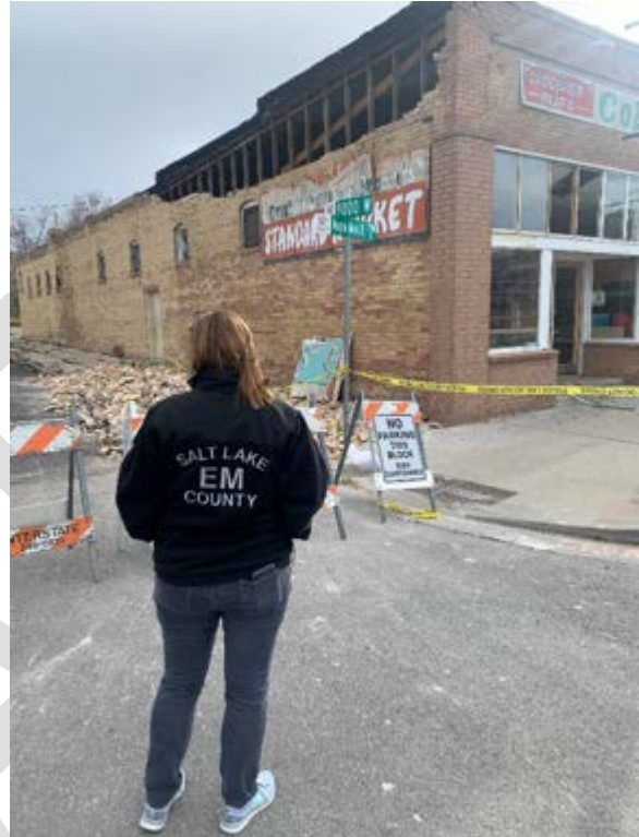
Figure 76: Effects of the 2020 Magna Earthquake
