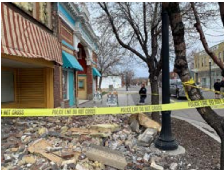
Figure 80: Damage Following the Magna Earthquake 101
