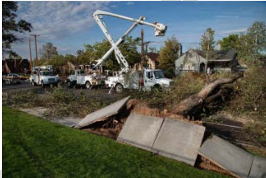
Figure 123: Damage from a High Wind Event in 2020 140
