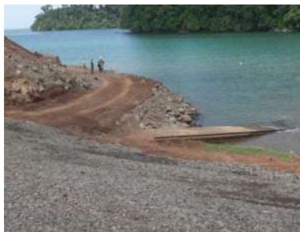
Figure 8.7. Site of APS SEABEE pier construction on Man-o-war bay base in 2009 (source: 2009 BIR After Action Report).
