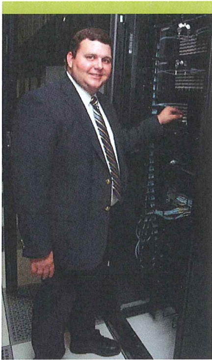
Jonathan Ouzts, RCDD, structured cabling project manager for CooperCraft Communications, checks the cable termination in the new Tift Medical Center 15,000-square-foot data center due to open this summer.
