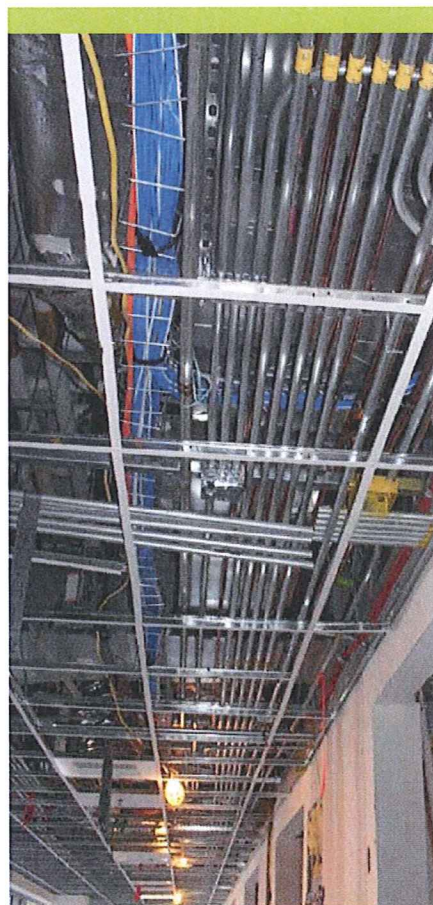
Horizontal cable in health care environments often share pathways with conduits containing gases and fluids.
