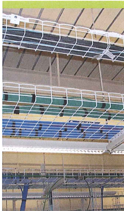
The TIA-1179 standard brings attention to separating cables by application, as shown here in the new Tifton Medical Center.
