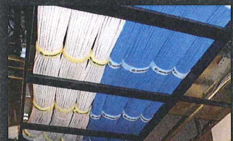
At Memorial Sloan-Kettering Cancer Center, the telecommunications cable is color coded blue for data and white for voice.
