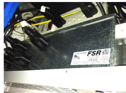
FSR CB-224 with fiber, copper and with an added power strip
