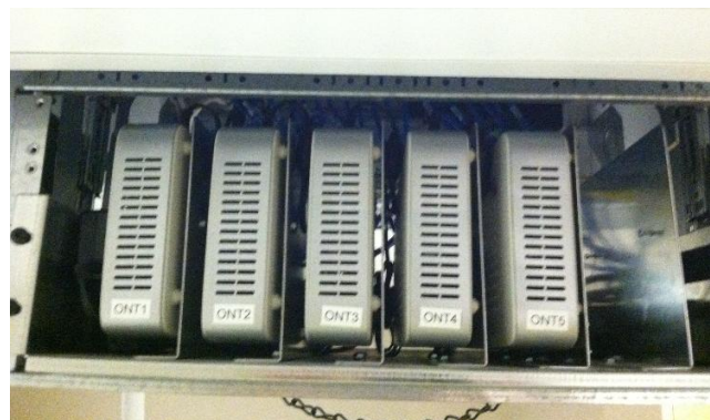
FSR CB-224 in a PON installation
