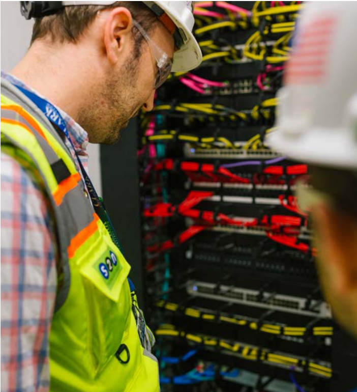
Ian Mitchell, RCDD, RTPM, LEED AP, Senior Project Manager for Systems Integration at S2N Technology Group, inspects the terminated Superior Essex category cable in one of the A/V rooms. The cable is color-coded for the different applications.
