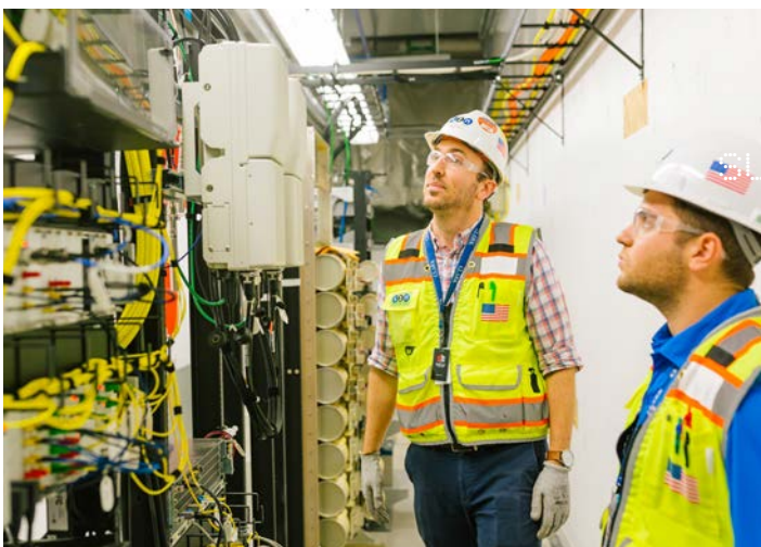
Ian Mitchell and Brody Pfeifer of S2N Technology Group inspect the cabling for the cellular distributed antenna system (DAS) and facility radio in the demarcation room.
