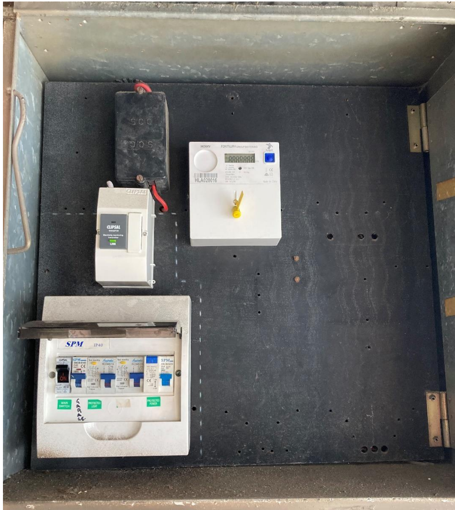
Photo 3: Photo of the switchboard:
