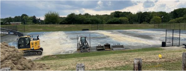
Summer tends to be a time of construction and renovation projects, and this year is no different. In addition to the resurfacing project on the outdoor tennis courts-which includes adding a pickleball court to the facility (above) -construction workers have been busy at the community park pond (below).
