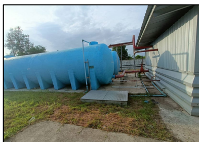
Water pipes directing water to the backup fire pump system
