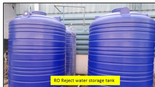
RO reject water is stored in storage tanks for reuse
