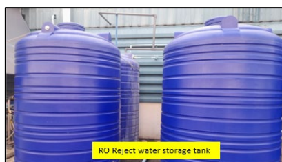
RO reject water are stored in storage tanks for reuse
