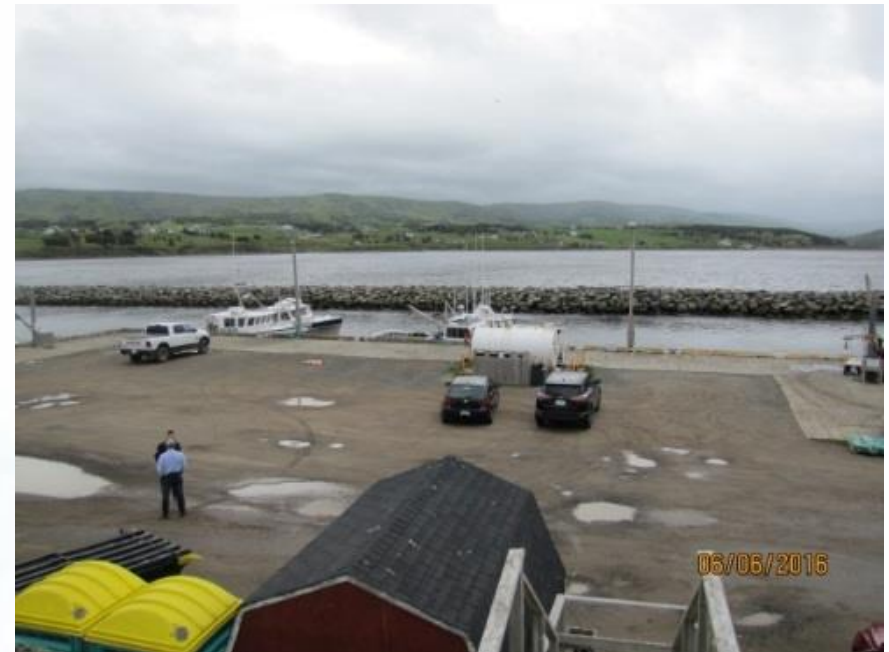
Margaree Harbour (2016): Wharf raised 0.7 metre Credit and source: Donald MacDonald, Fisheries and Oceans Canada, 2016
