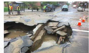
Flood damage from water pipe puncture.
