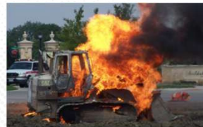
Accident resulting from compromised gas main.
