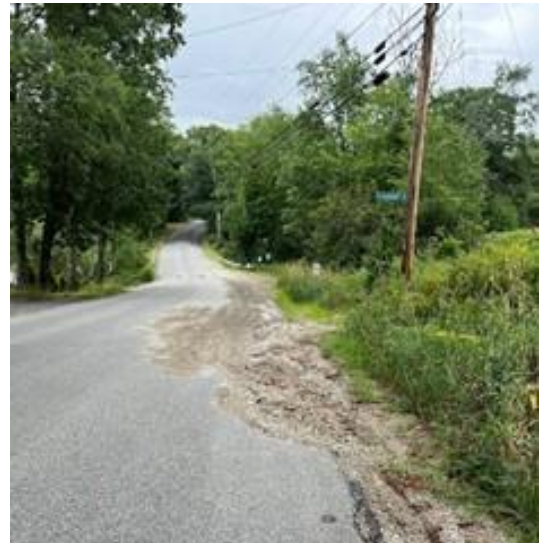
Sediment accumulation of road due to erosion, uphill from the Barnstead Boat Ramp.
