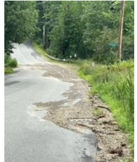
The eroding road shoulder leading to the North Barnstead Rd boat ramp.
