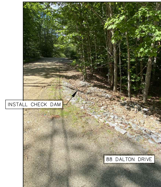
DALTON DRIVE DRAINAGE SWALE (WEST SIDE OF ROAD)
