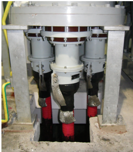
SSC140-SF terminations installed in a GIS.
