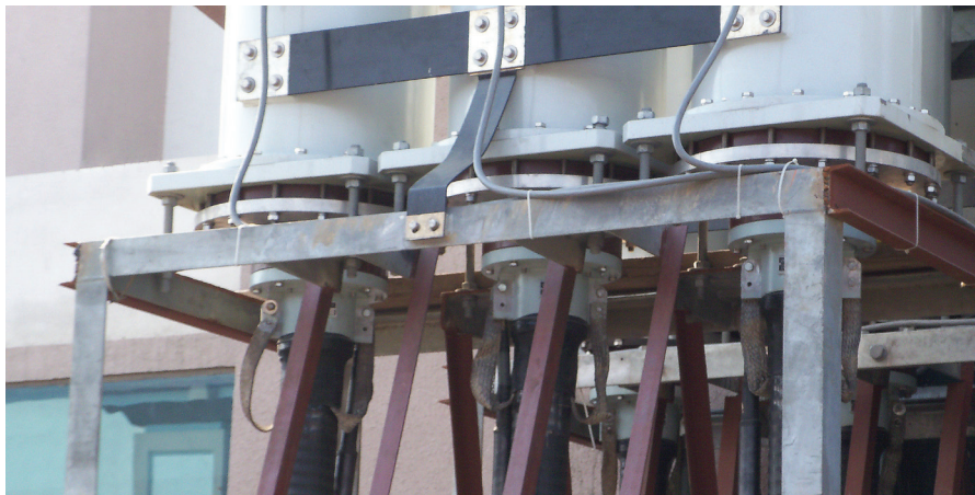
PATR140-SF terminations installed in a GIS.
