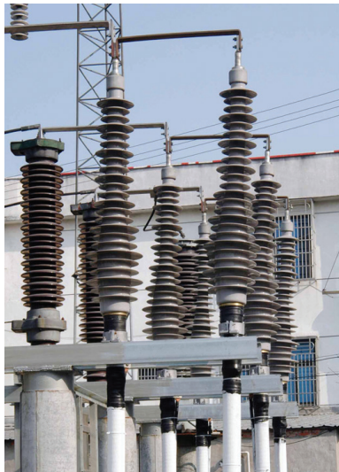
Dry type outdoor termination in a substation application.
