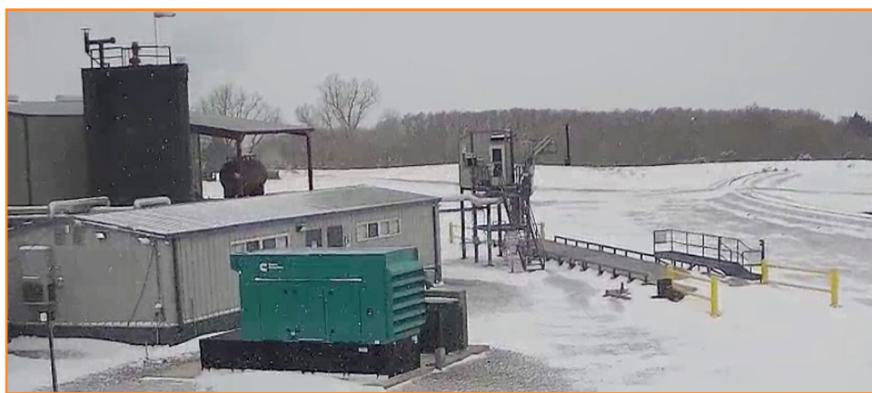
A new generator was installed at the Clinton, OK facility in December.
