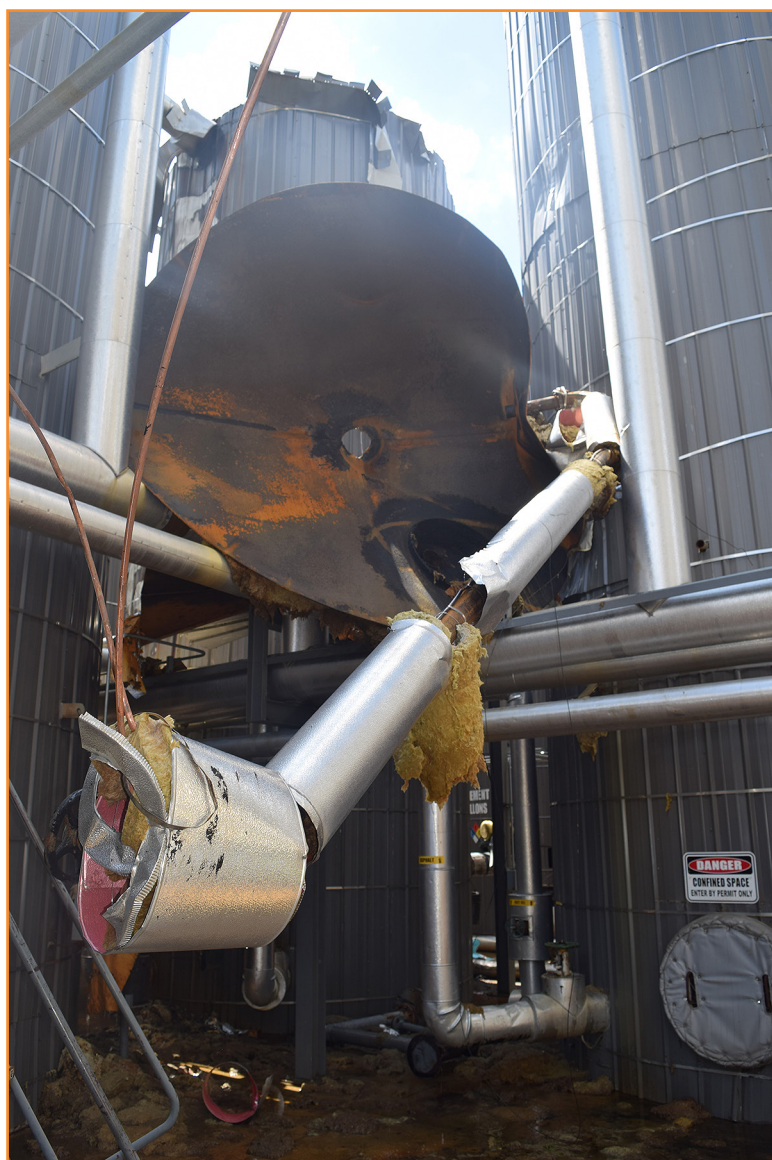
Some of the damage caused at the plant.
