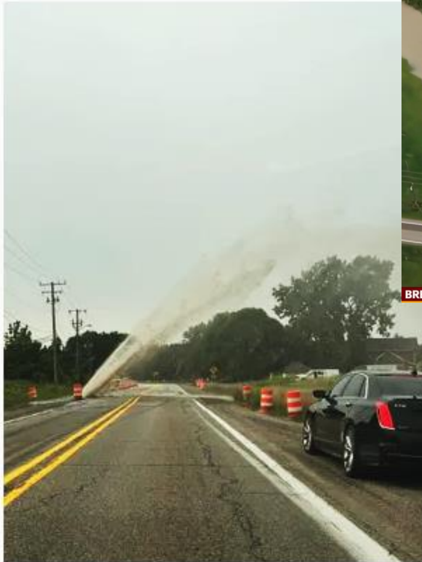
A water main break is pictured near the intersection of 22 Mile Road and Romeo Plank on Tuesday, Aug. 1, 2023. Provided By Andrew Plunkett
