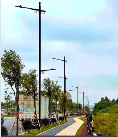
Guangzhou Xintang NB Street Light Project
