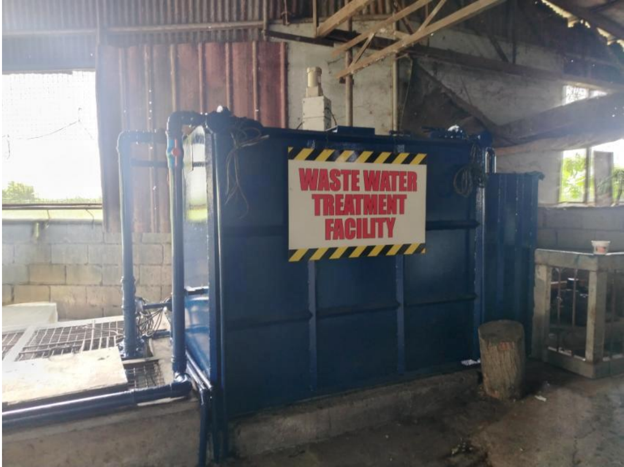
Final project installation at Kerith Brooks Trading
