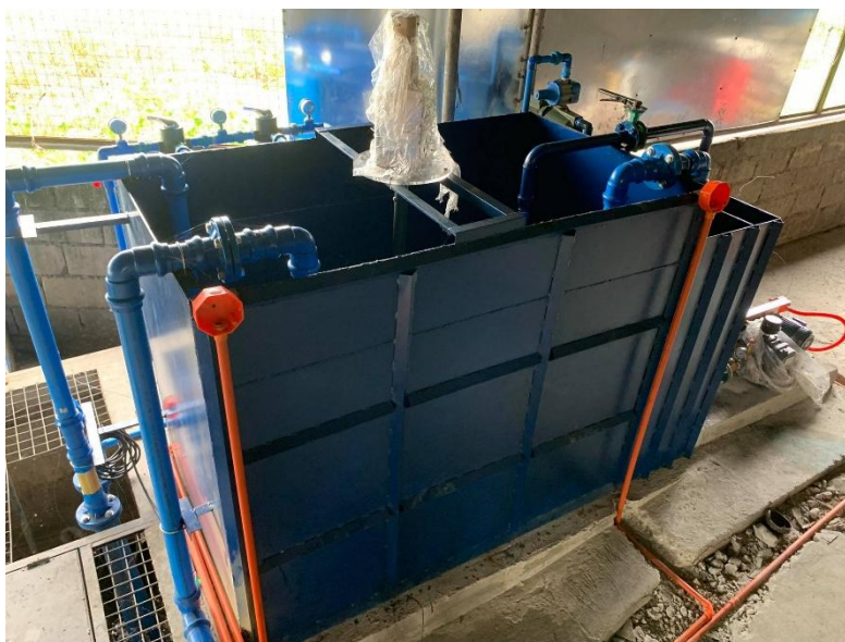
Completed BioCube™ system at Kerith Brooks Trading
