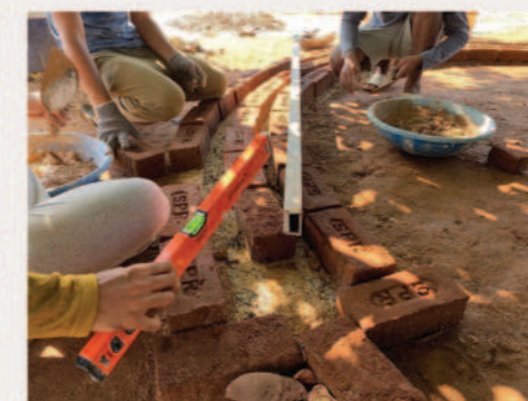
Bricks placed on the base structure on both the sides using mud mortar
