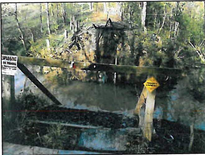
Bridge area prior to removal of bridge - looking west. Bridge was knocked down and partially carried away by flood waters in 2011.
