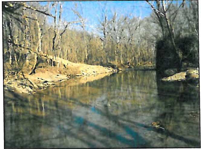
Bridge area March 2012 after removal of bridge and grading and stabilization of west stream bank.
