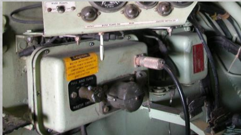
Master Switch Box & Fuse Box
