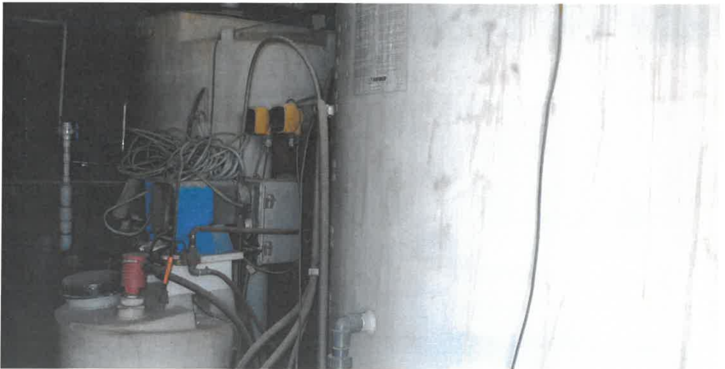
Photograph 10 Storage tanks for acid in north building
