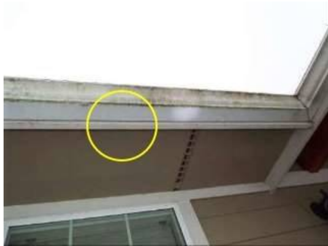
Photo 31-2 Water leaking behind gutter
