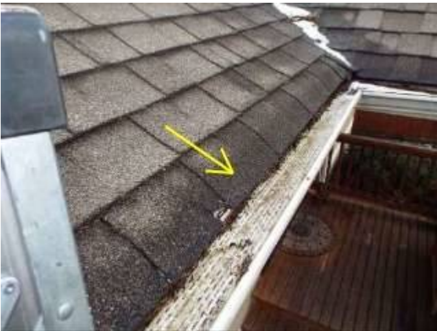
Photo 32-1 Debris in front of house
