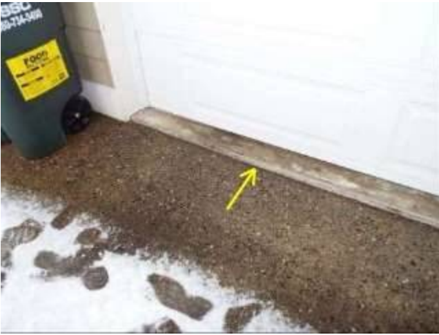
Photo 23-1 Lip in front of garage
