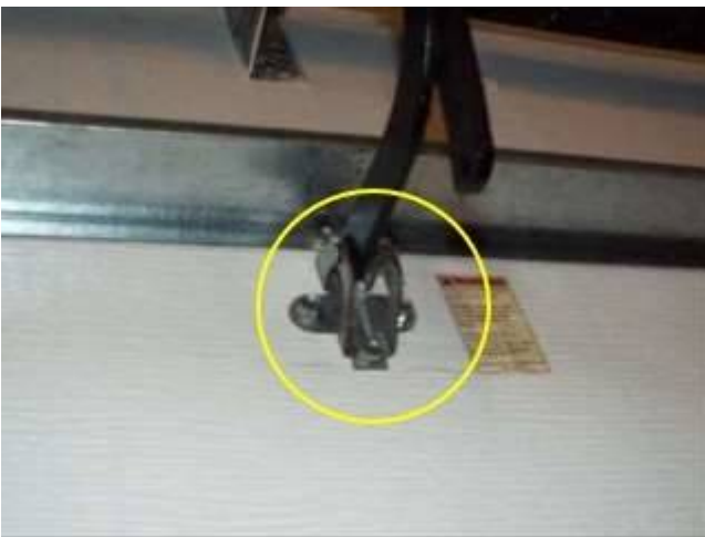
Photo 22-1 Bracket pulling and cracking garage door
