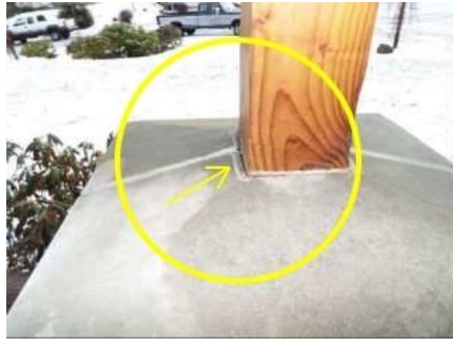
Photo 10-2 Front porch, pooling water at base
