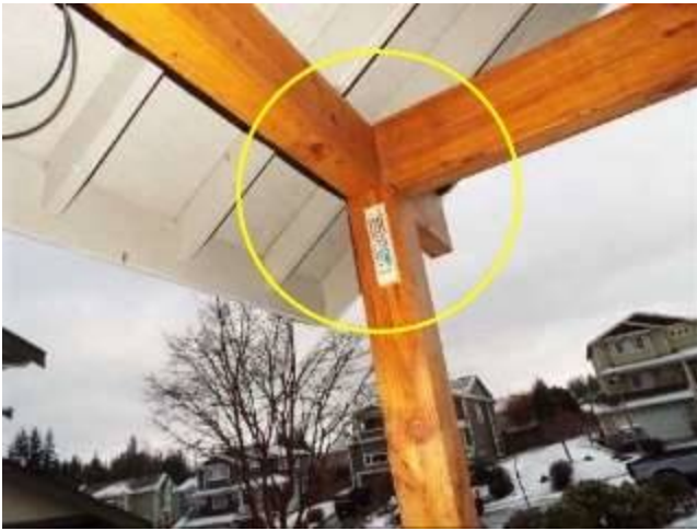
Photo 10-1 Front porch, missing brackets
