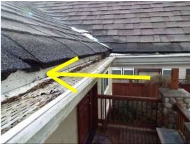
Photo 31-1 Lack of flashing from roof to gutter
