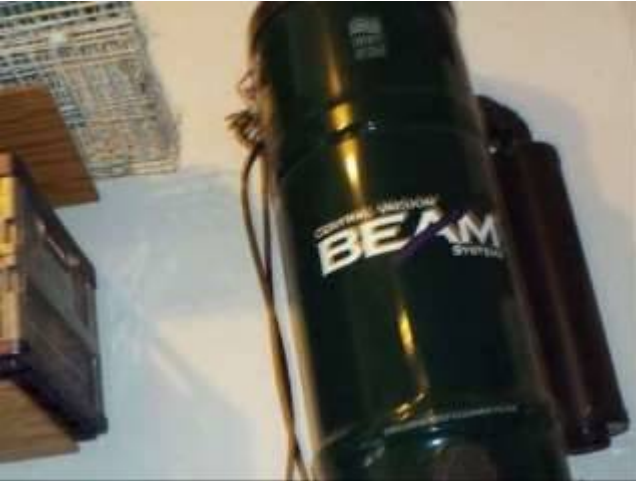
Photo 24-1 Main unit located in garage
