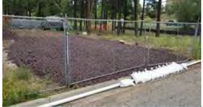
Rock and cinder track out pads prevent sedimentation to streets adjacent to the project location.
