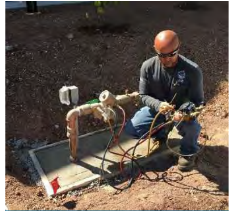
Staff performing a backflow test.
