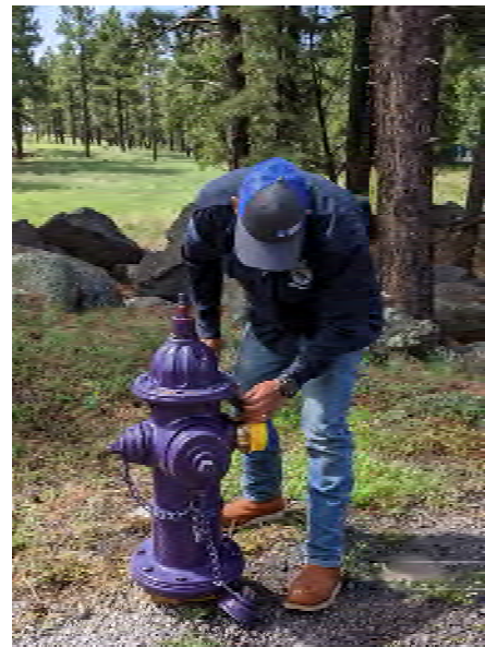
Crew member installing a smart field device to capture real-time pressures in the reclamation distribution system.
