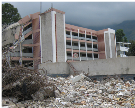
Canado-Haitian Secondary School The debris are from the northern part of the building while the eastern part is being demolished.
