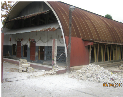
One of the two curved roof building after the earthquake
