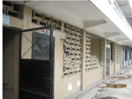
This is the first concrete building constructed in Pope Jean XXIII school. It needs repairs.
