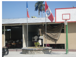
Two new classrooms at the Canado Secondary School as a consequence of the 2010 earthquake
