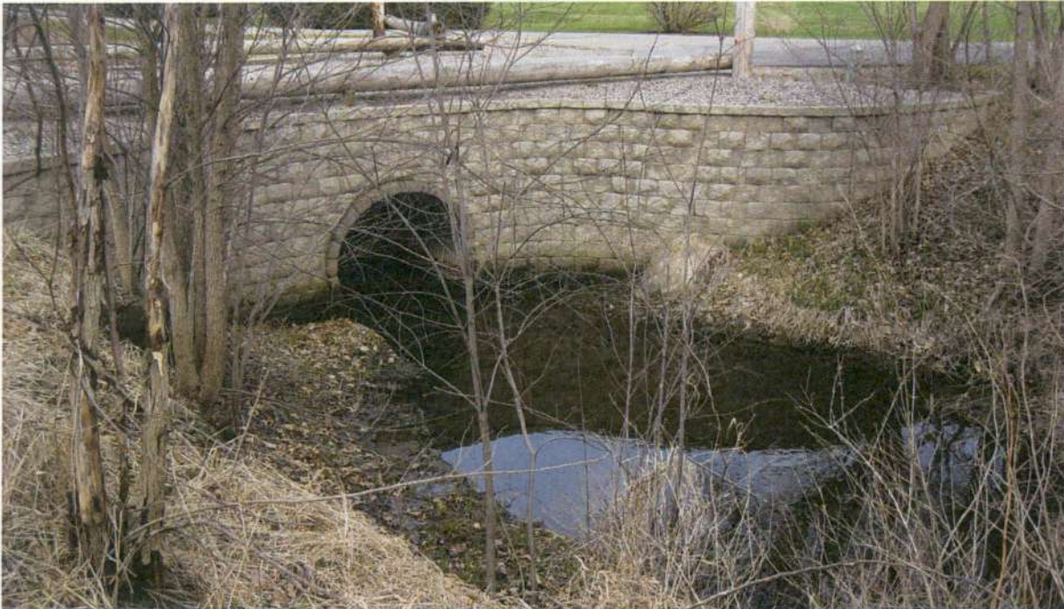
Picture No. 17 shows the eastern downstream end of the 66-inch CSP culvert under Meadow Valley. Picture is taken looking northwest.
