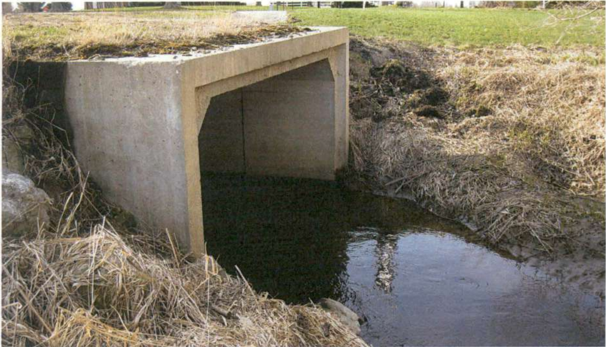
Picture No. 14 shows the western upstream end of the 8-foot by 12-foot concrete box culvert crossing under Patterson Ave.
