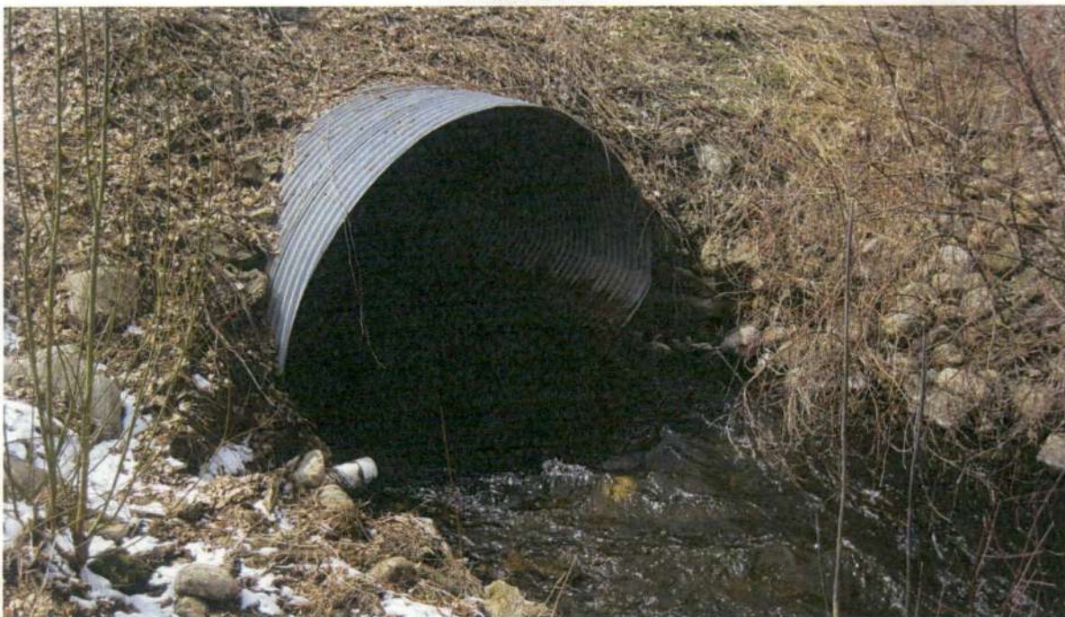
Picture No. 7 is looking at the east downstream end of the 7.5-foot by 11.5-foot elliptical CSP culvert crossing under Noffke Road. Picture is taken looking towards the west.
