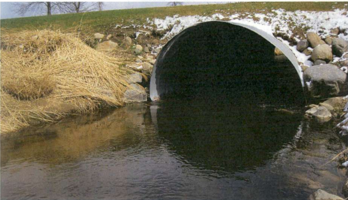
Picture No. 6 is looking east at the southern upstream end of the 8-foot by 12-foot CSP culvert under Duncan Lake Road.
