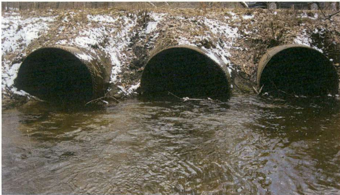
Picture No. 2 shows the upstream north end of the three steel culverts. The culvert on the far right of the picture (east culvert) has accumulated approximately 12 inches of sediment.
