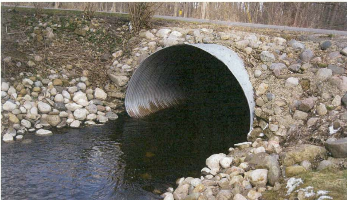
Picture No. 8 is the western upstream end of the 7.5-foot by 11.5 foot elliptical CSP culvert. There is slight distortion near the springline of the pipe. Picture is taken looking towards the northeast.
