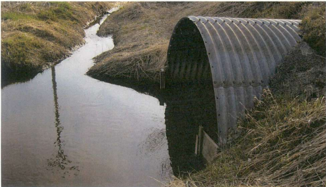
Picture No. 12 shows the upstream northern end of the 9-foot by 12.5-foot arch CSP culvert crossing under 100 th Street.
