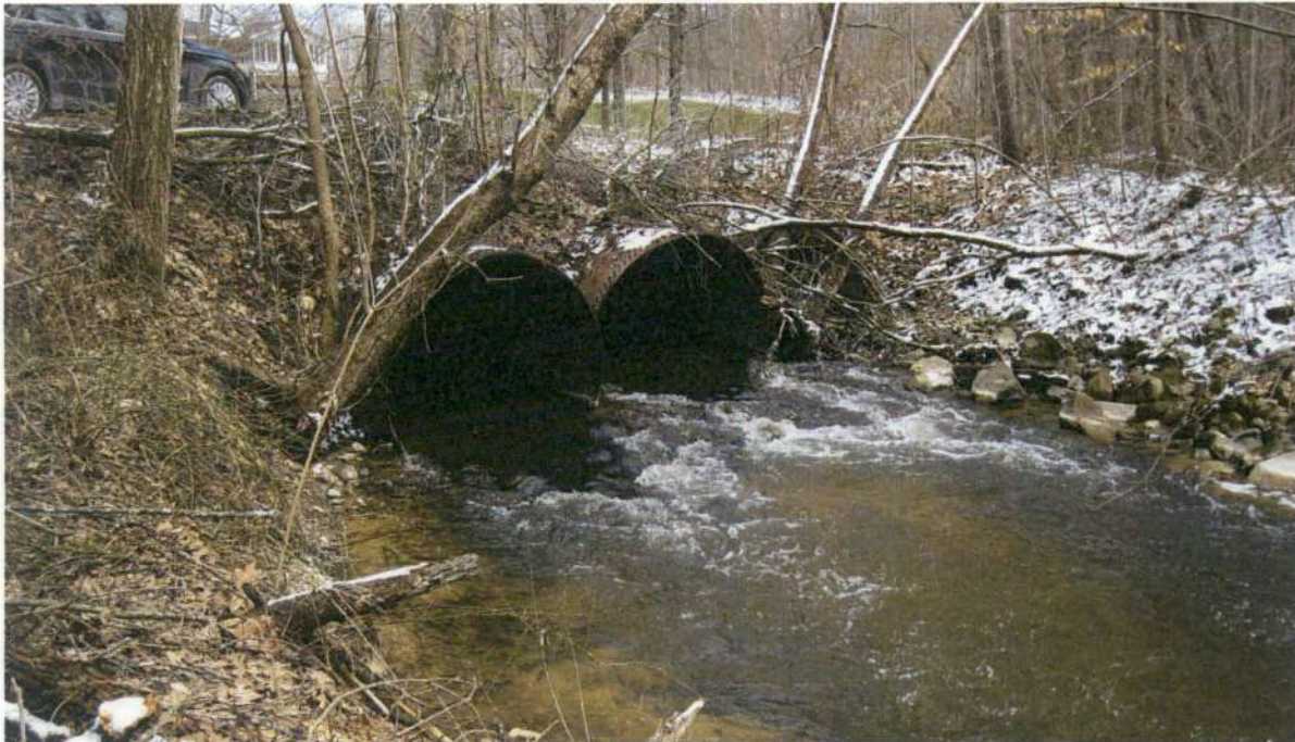
Picture No. 1 shows the southern end of the three steel culverts under Garbow Road. Dead trees have fallen across this outlet end of the eastern culvert.
