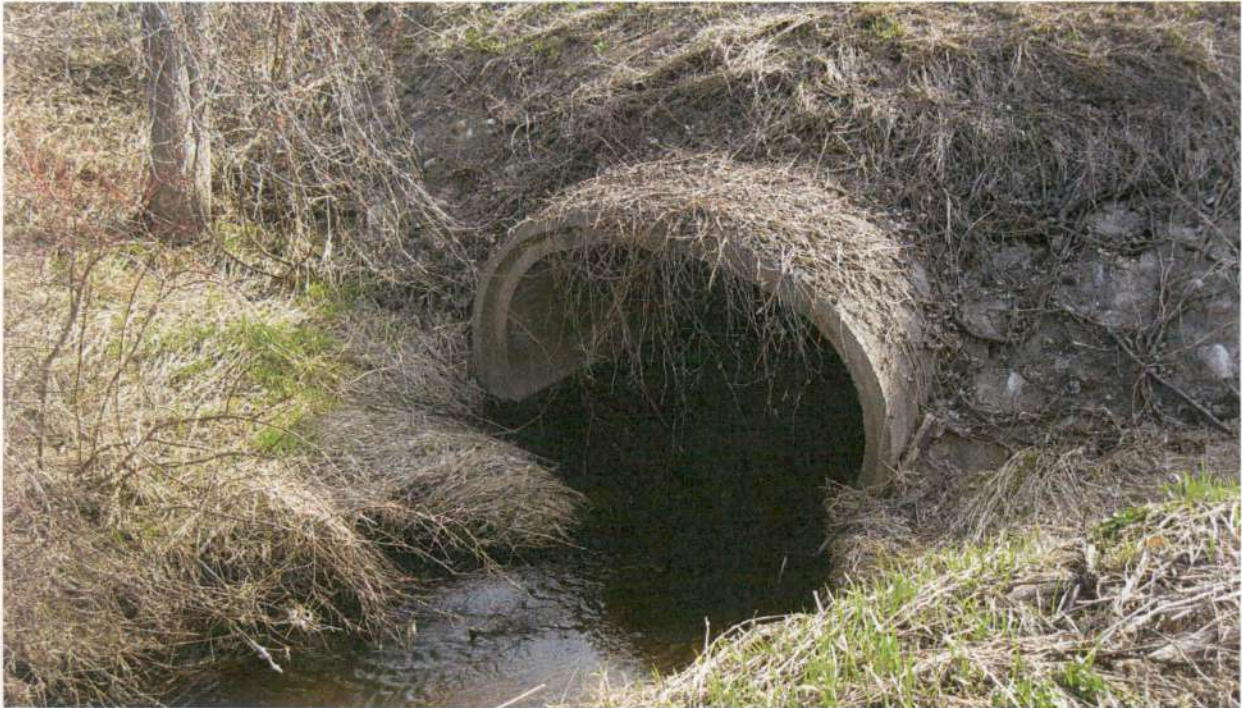
Picture No. 16 shows the upstream western end of the 5-foot by 9-foot elliptical RCP culvert crossing under East Paris Ave.
