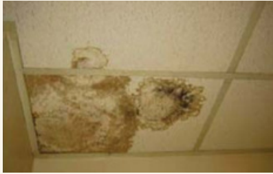
Figure 3 - Water Leak in a Garrison Facility at Walter Reed (courtesy US Army)
