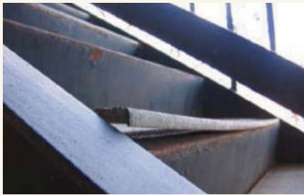
Figure 2 - Stair Tread Problem, a tripping Hazard (courtesy US Army)
