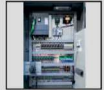
• Fanuc/Mitsubishi Drivers and Schneider Electrical System
