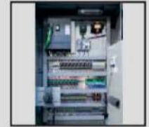
• Fanuc/Mitsubishi Drivers and Schneider Electrical System
