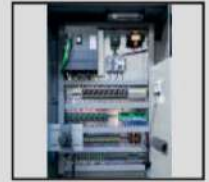
• Fanuc/Mitsubishi Drivers and Schneider Electrical System
