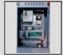
• Syntec & Fanuc Drivers and Schneider Electrical System
