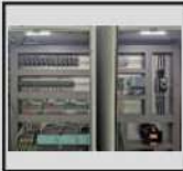
• FANUC/Mitsubishi Drivers and Schneider Electric System
