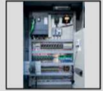
• Fanuc/Mitsubishi Drivers and Schneider Electrical System
