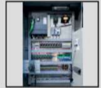
• Fanuc/Mitsubishi Drivers and Schneider Electrical System
