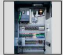
• Fanuc/Mitsubishi Drivers and Schneider Electrical System
