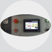
PLC Kontrol Panel PLC Control Panel
