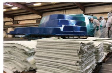
Four layers of fiberglass, comprised of chopped strand mat and 36 ounce mat, are applied.
