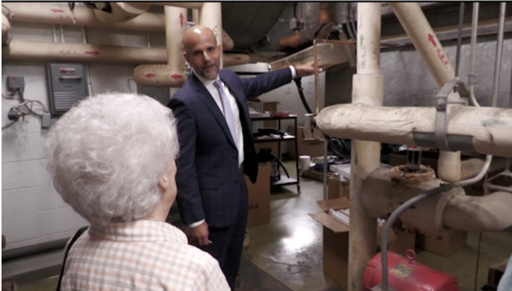
Former North Penn High School Principal Pete Nicholson, now a district administrator for secondary education and renovations, shows residents aging infrastructure and equipment that could be replaced during potential NPHS renovations. (Photo courtesy of NPSD)
