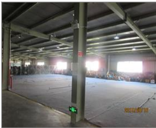
Photo of fire safety equipment Evacuation sign.JPG
