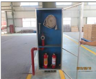
Photo of fire safety equipment Fire hydrant and extinguishers.JPG
