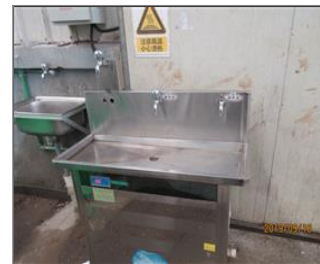
Photo of the sanitary facilities Drinking water.JPG
