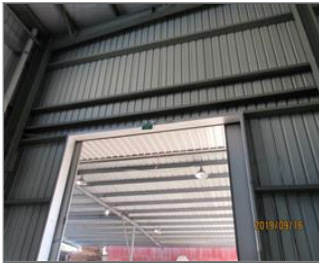
Photo of fire safety equipment Emergency exit sign and light.JPG
