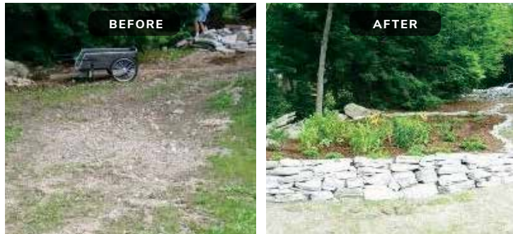
This rain garden (right) will help prevent erosion and reduce the amount of surface water running downhill and into the lake.
