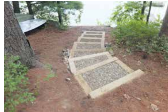
Infiltration steps slow down and soak up runoff water.
