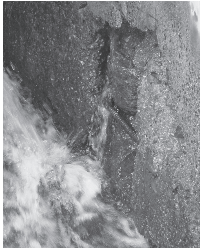
Spalling produced by channeling, west concrete pier
