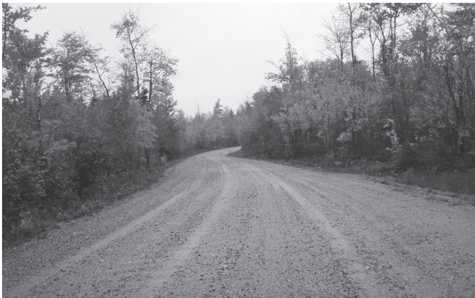
A properly contoured gravel road reduces polluted run-off.
