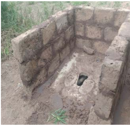
Construction of latrines is underway, signaling the community's prioritization of proper sanitation and hygiene.
