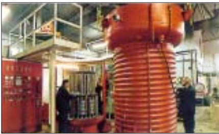
Ion nitriding plant
