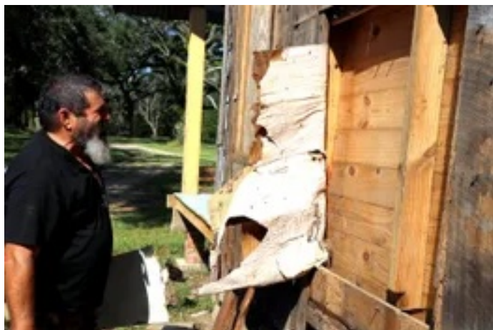
Cardboard was used for both insulation and wallpaper. (photo by Wanda Carole Wrinkle Ford)
