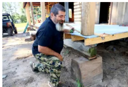
Ricky Dowden shows off pier and support beam. (photo by Wanda Carole Wrinkle Ford)
