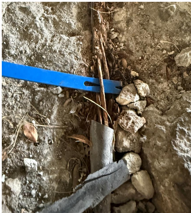
Photo 4: Failed Tendon Test
