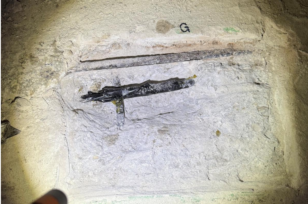
Photo 7: Good Tendon; Greased and Wrapped
