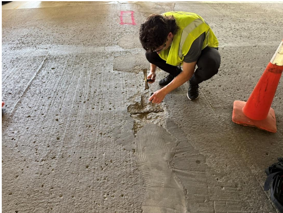
Photo 2: Tendon Exposed at Concrete Spall
