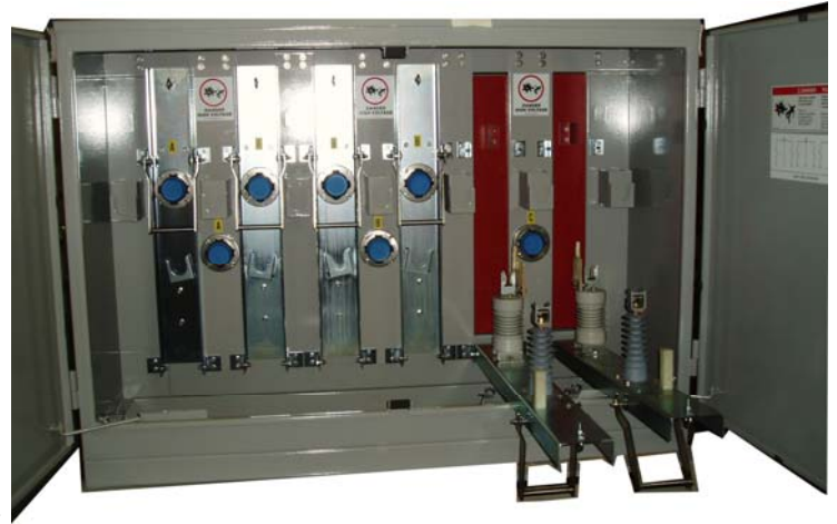
Figure 1. 15 kV 200 A Fuse Gear with (2) Fused Ways
