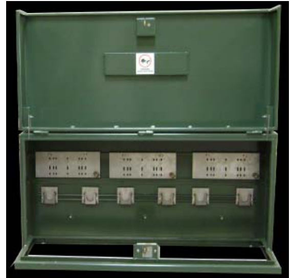
Figure 1. Standard Termination cabinet.
