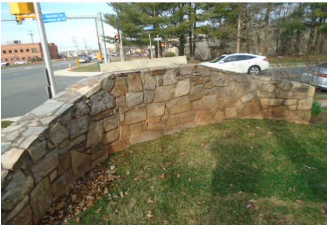
Stone faced feature at entrance is a long lasting component that can be kept in good repair with spot repairs.
