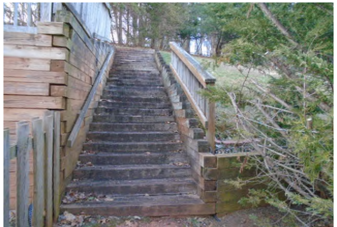
Association is only responsible for the retaining walls on each side of the staircase. All other retaining walls are owner responsibility. Stairs are a long lasting items if maintained and repaired as needed.
