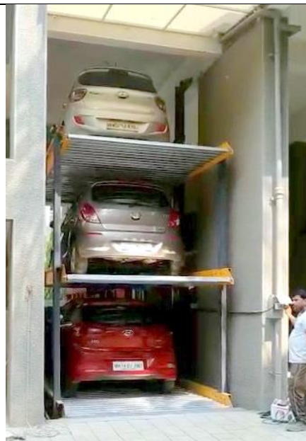
G-2 Stack Parking System (Independent, 3cars/System), Client: Vandanshree, Gokhale Constructions, Pune
