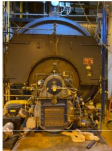
Butler Boiler #3 Front view
