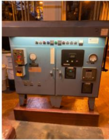
Butler Boiler #3 Control panel
