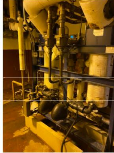
Butler Instantaneous Hot Water Heater with Leaking Flange
