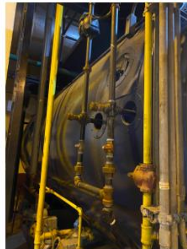
Butler Boiler #3 Left side
