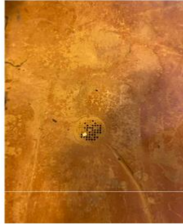
Figure #: Butler Floor drainage clog
