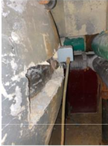
Butler Condensate Tank Missing insulation
