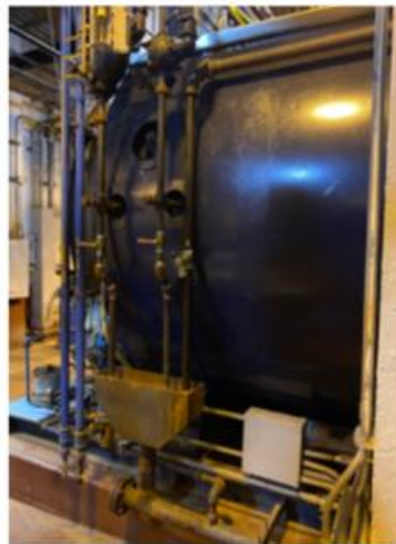
Butler Boiler #3 Right side clogged overflow trough
