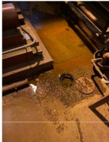
Butler Floor drainage clog
