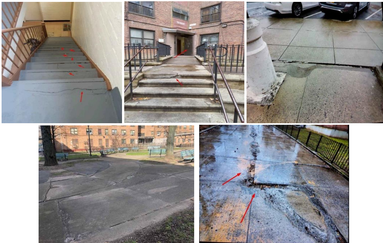
Recent photographs from Monitor field reports provided to NYCHA (from left to right): a cracked staircase; cracked steps; a cracked sidewalk; a damaged courtyard; and a damaged sidewalk.
